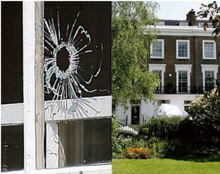
Point of impact: A bullet hole in one of the windows of the flat (left), Exclusive residence: The £2million flat in Markham Square
